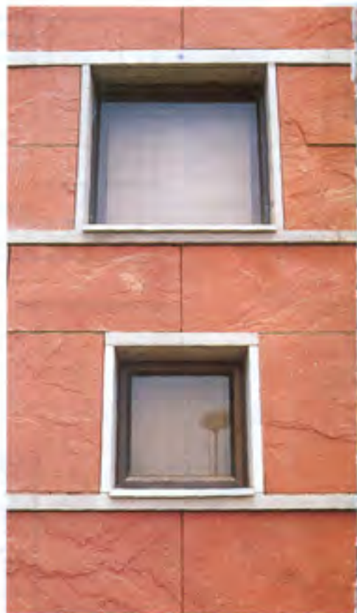
External cladding of rough-split red sandstone dry-hung with pre-cast terrazzo jambs and cills around windows.
